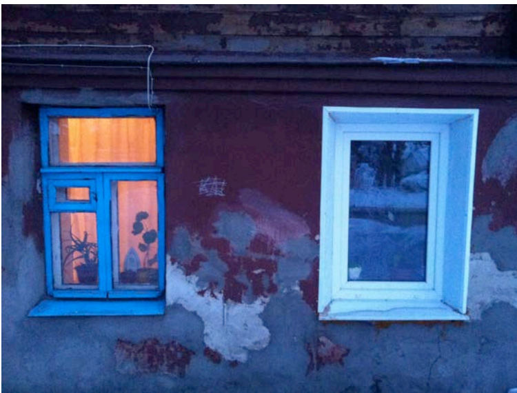
picture 5 – View of window frames on the ground floor of a wooden house. Please note that bad restoration attempts or makeshift maintenance measures carried out to increase the functional and energy saving performances of the buildings can actually jeopardize aesthetic and cultural aspects of the house, without enhancing its functional aspects. The PVC window frame in the picture lacks the functional devices of the original wooden frame, namely the multiple-opening system, hence reducing the energy saving upgrade provided by the new window frame.
